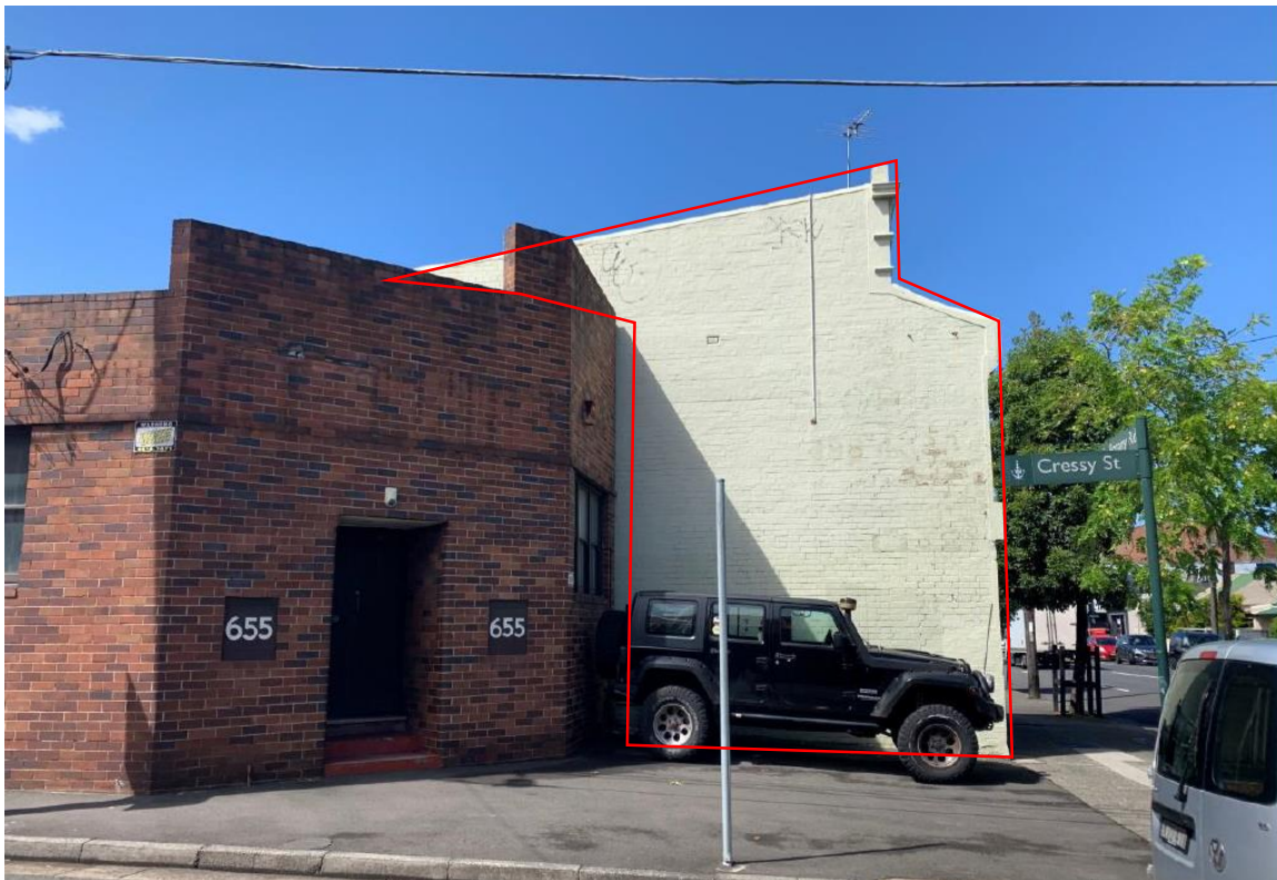
Figure 6: Photo showing the existing northern elevation of the existing terrace building, as seen from Cressy Street. The existing terrace building retains the original setback along Botany Road.
